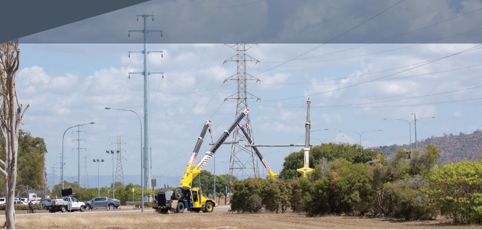
Replacing the ageing Garbutt to Alan Sherriff transmission line to maintain a safe and reliable electricity supply to the Townsville region.
