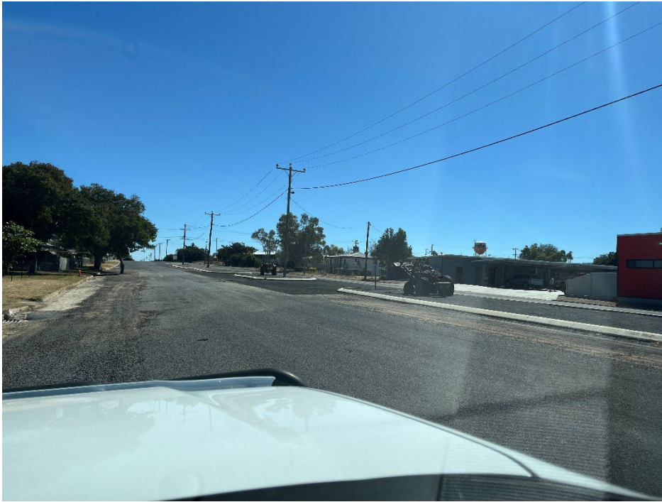
Figure 3.2: Bitumen condition of a road in the Richmond township
