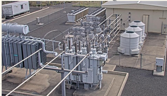
Reactive plant – SVC
