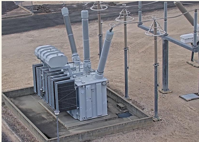
Reactive plant - Reactor
