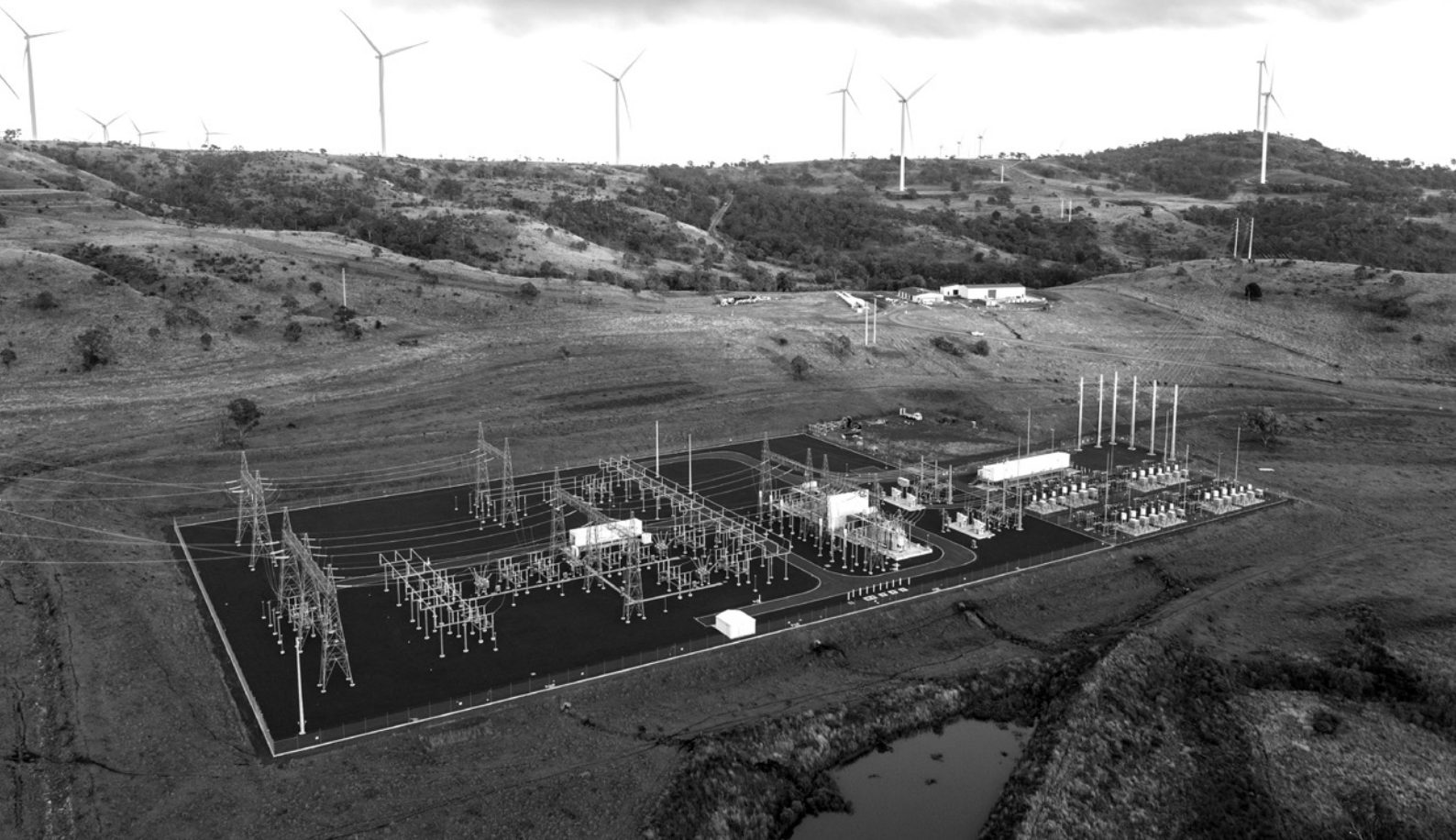
Aerial view of Powerlink's substation in front of wind turbines from the Coopers Gap Wind Farm.
